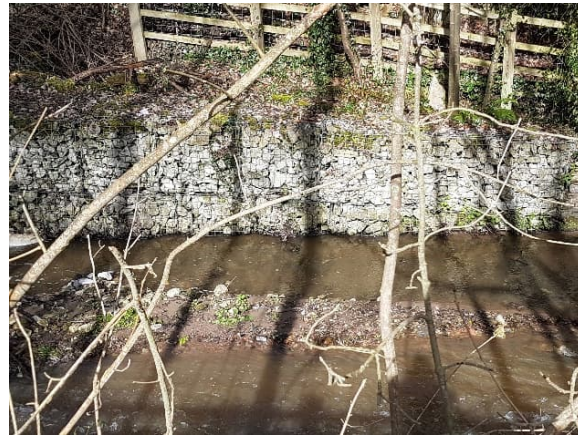
Channel is over-wide at the culvert outlet and continues to be over-wide through the modified reach where gabion baskets line both banks downstream of the A55 culvert.
