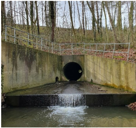
A55 culvert – view looking upstream. Culvert is perched above the natural stream bed.
