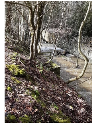
View looking upstream towards the A55 culvert outlet showing the transition from the modified reach with gabion basket bank reinforcement.
